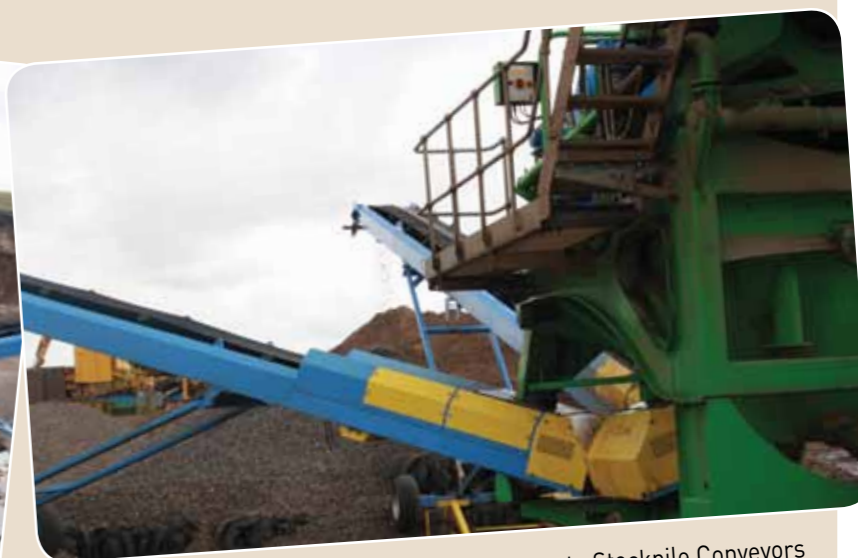
Malcolm's Aggregate Stockpile Conveyors
